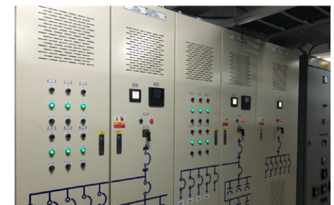
▲ Smart Electricity Control System
